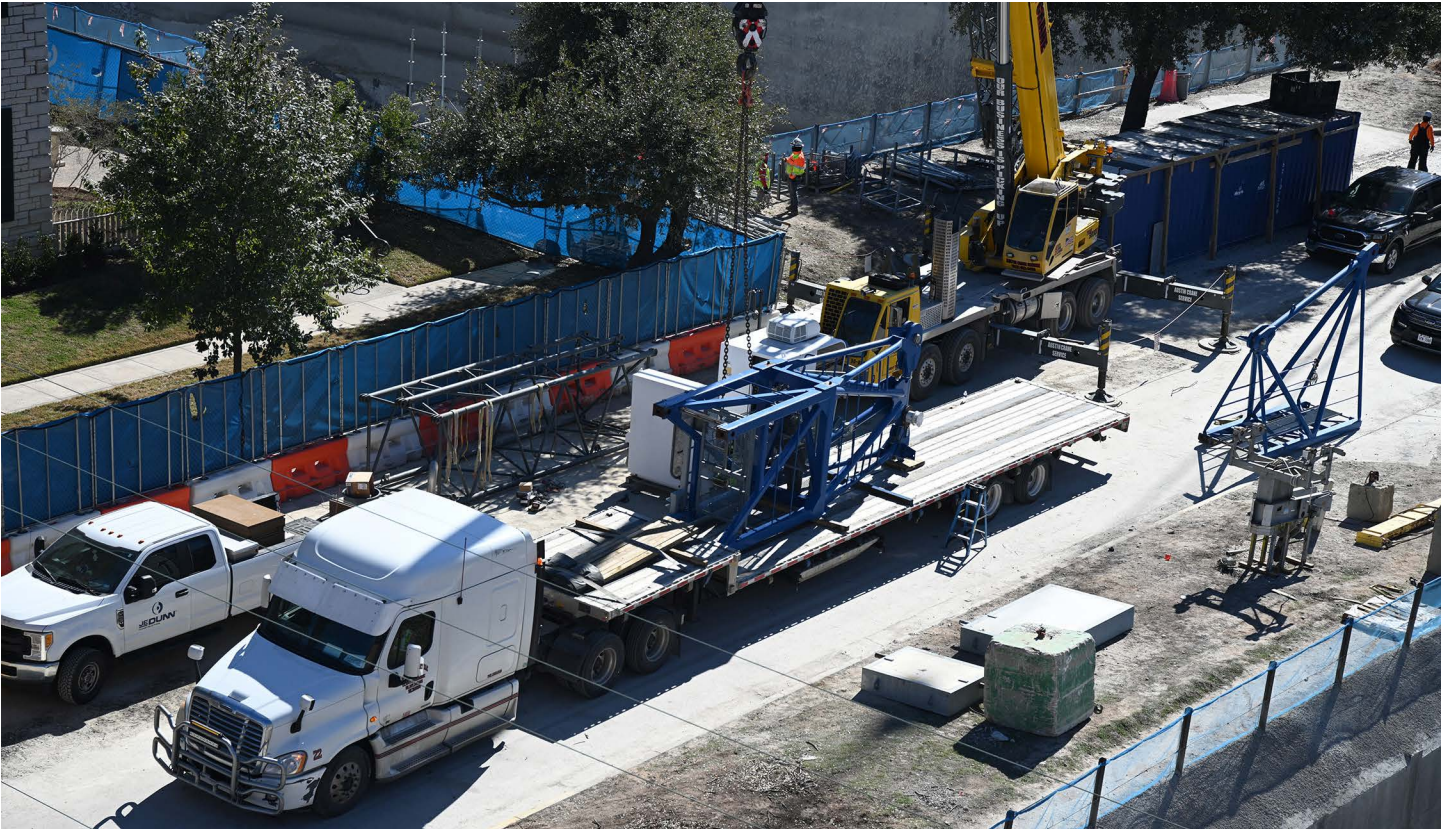
The JE Dunn Assemble and Dismantle team prepare to unload a section of the 1501 Lavaca tower crane from a truck.
