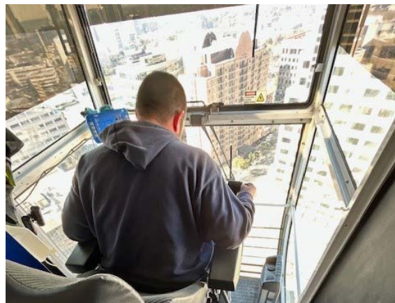
JE Dunn Crane Operator Gerrard Hennessy pilots the 1501 Lavaca tower crane high above the Capitol Complex.
