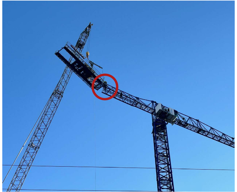
A member of the JE Dunn's AD team (in the red circle) connects a section of the jib held by the assembly crane.
