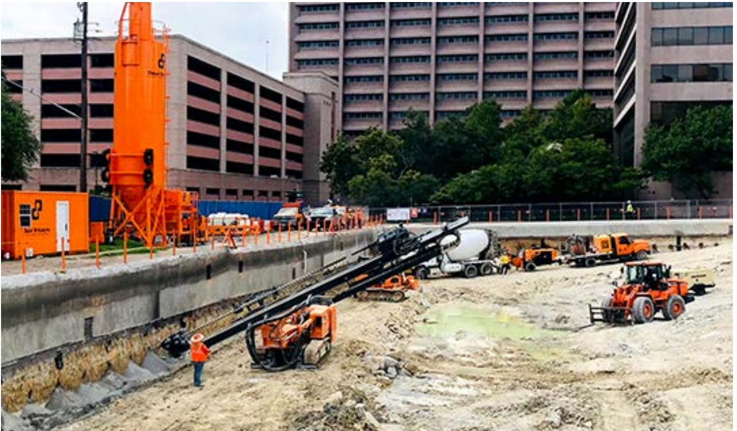
The team installs anchors into the wall face on Phase II. A shotcrete pump at ground level is readied for the next step in the process.
