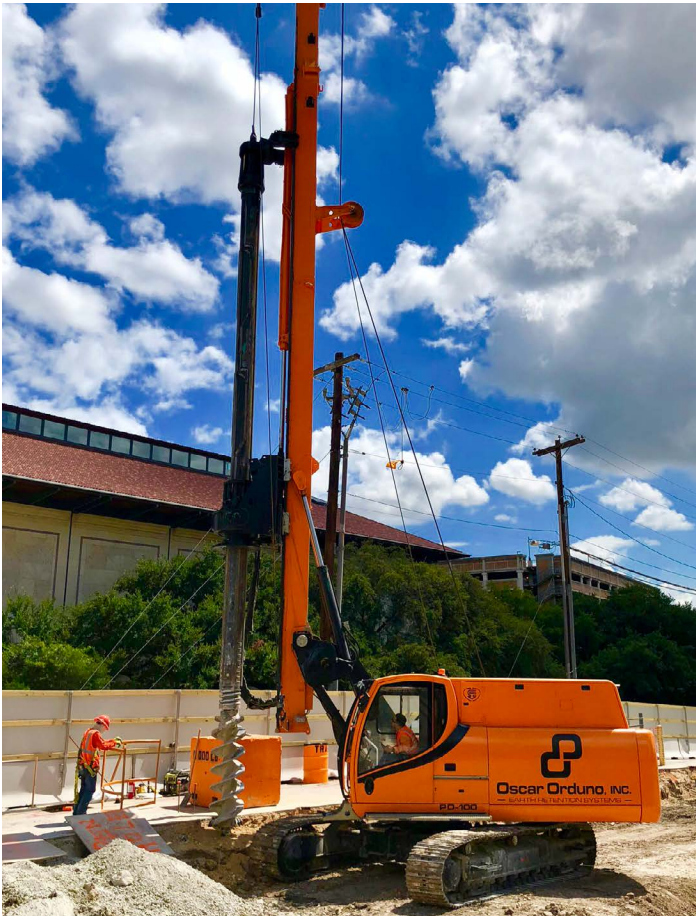
An Oscar Orduno team member operates a drill rig and pier drill while another team member helps monitor the progress.
